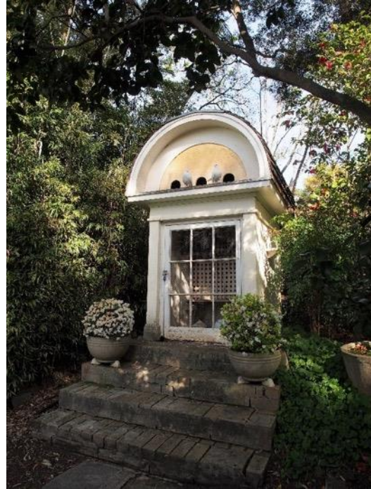
Figure 7.8h. The pigeon house in 2019 after conservation work, including a new timber shingle roof and re-gilding of the tympanum.
